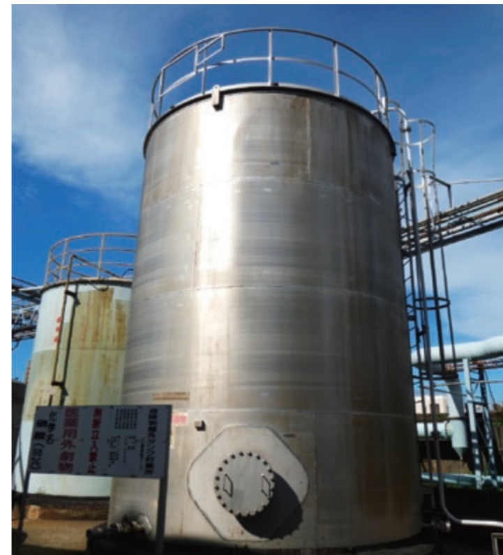
Nitric acid tank (SN-1)
