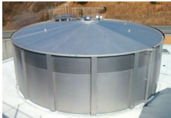
Water supply plant (304, 316, SUS329J4L)
