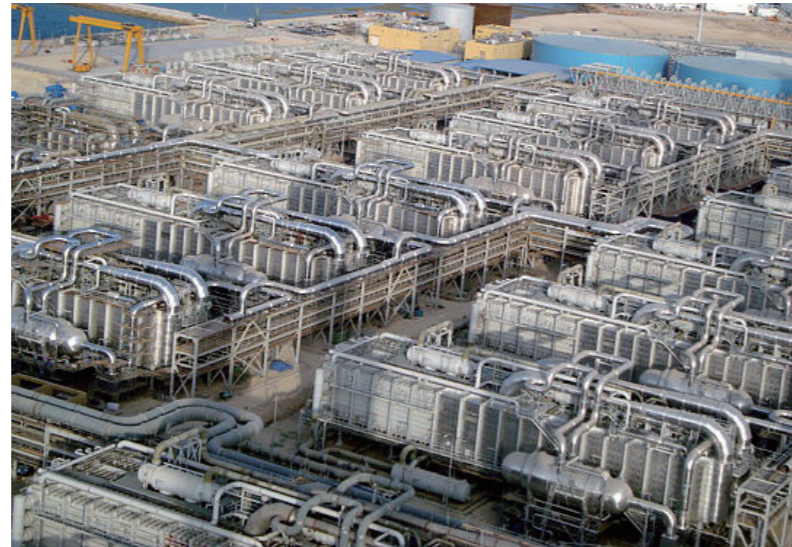
Desalination Plant (S32101, S82122, NSSC2120, S32304, S31803, S32205, S32750, S31254, NSSC270)
