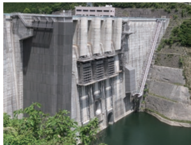
Dam intake tower, High-pressure gate (SUS304, SUS821L1, NSSC2120, SUS316L, SUS323L)
