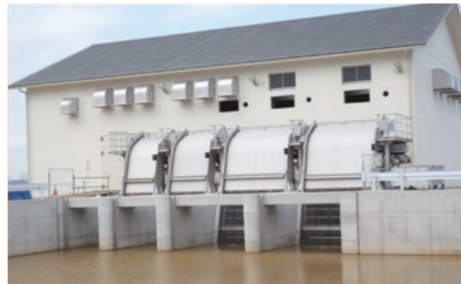
Drainage pump station, Dust remover (SUS304, SUS821L1, NSSC2120, SUS316L, SUS323L)
